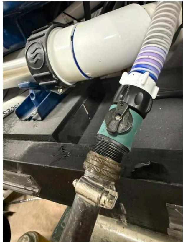
Figure 2. Valve is open
